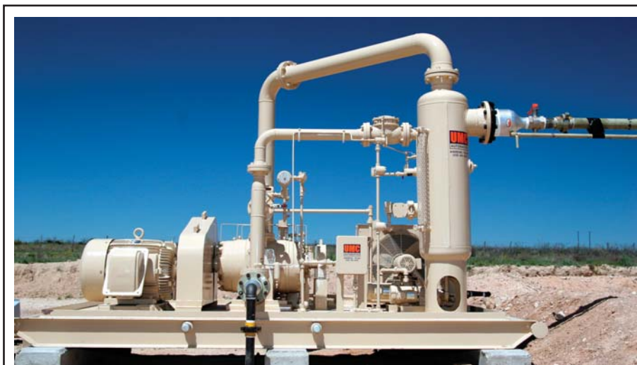
Murex Petroleum Corp. is using vapor recovery technology in developing horizontal Bakken oil wells in the Williston Basin to capture the rich gas streams that flash from the tanks of newly completed Bakken wells. The company has additional VRU installations that recover gas vapors from sour oil wells with high H 2 S content.
